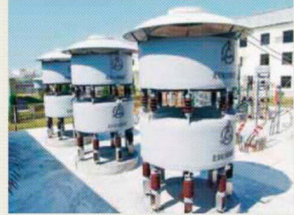
Thyristor Controlled Reactor
